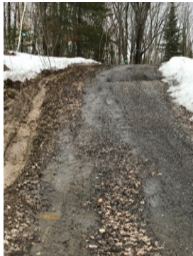
Sink hole on Morningside Drive
